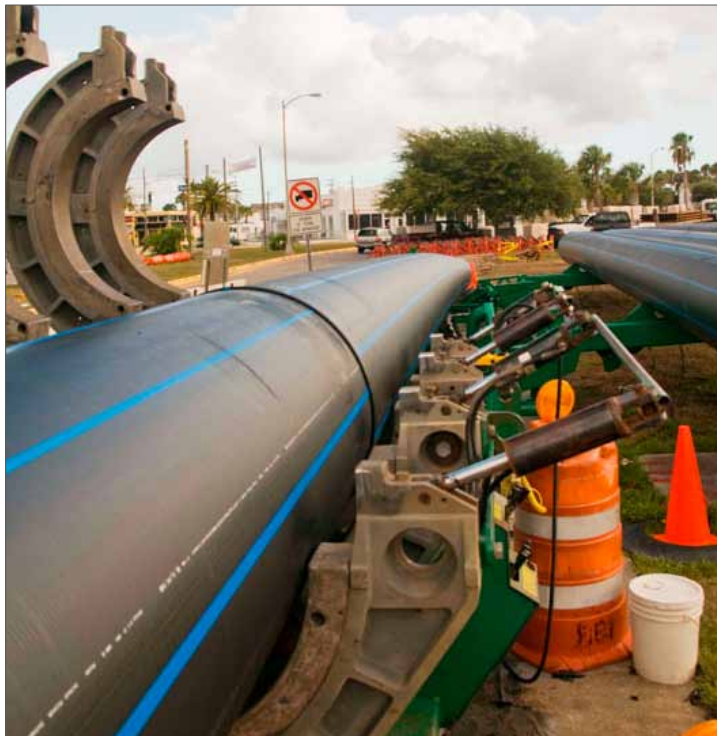
After a fusion joint was cooled, heavy machinery pulled the pipe through to be in position for the next fusion joint.
