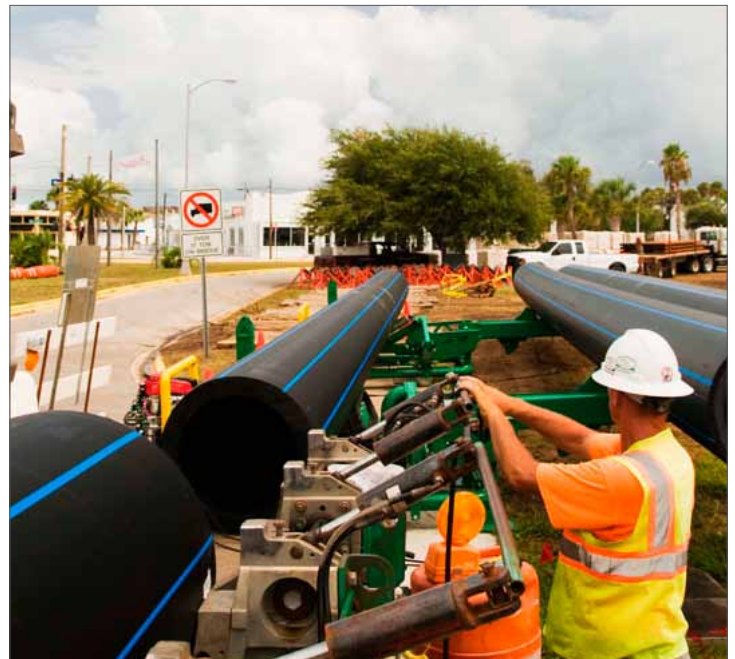
A stick of pipe is dispensed into the powered rollers of the MegaMc PolyHorse. The length of fused pipe has been pulled and is ready for the next 50-foot stick of pipe to be fused onto the length.
